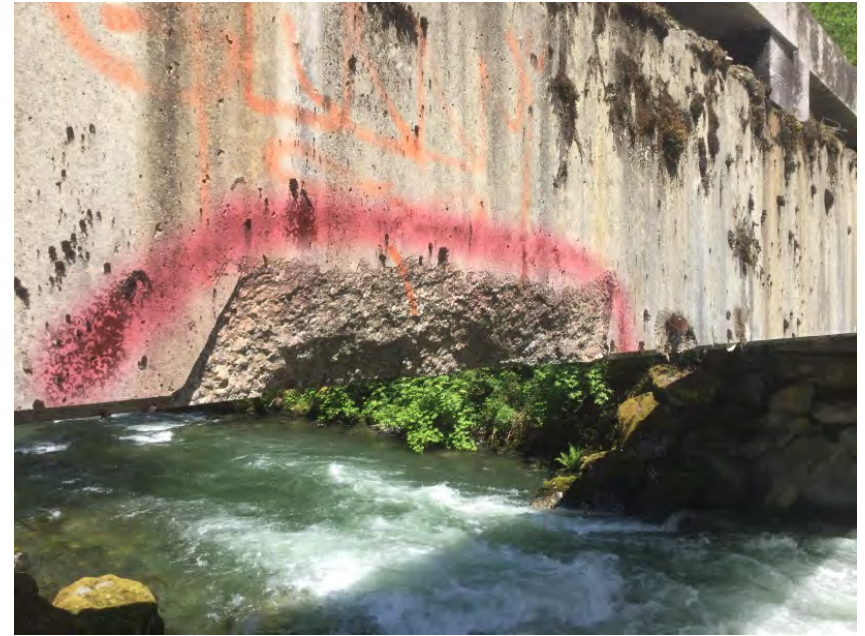
Upstream left bank girder damage
